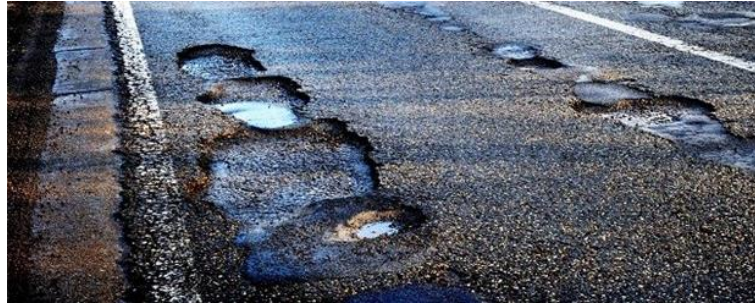
Figure 30: Potholes in road [38]
