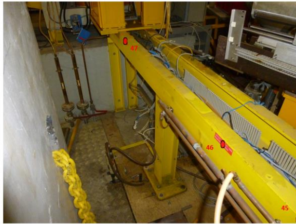
Figure 61 - Beam tube support structure from beam exit to switching magnet
