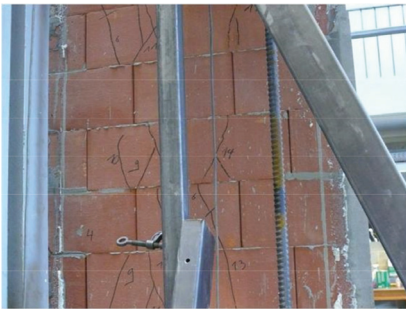
Figure 6. Cracking in the wall.
