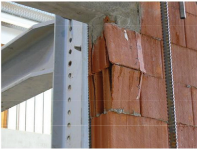
Figure 5. Failure at lintel support.
