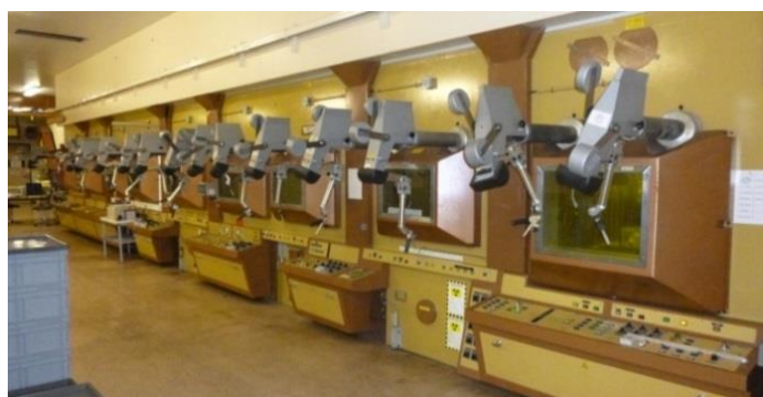
Figure 1: hot cells in the chemical zone
