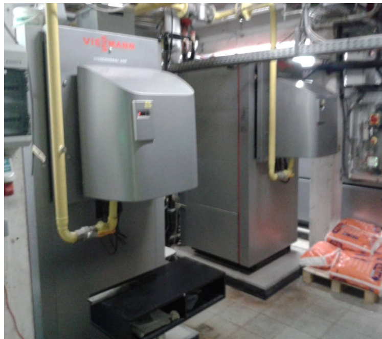
Figuur 15 Condenserende gasketels in cascade Demerhof
