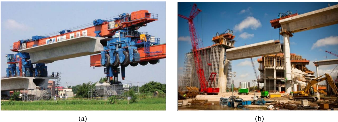
Figure 13: Execution examples full span construction technique: (a) with launchin cantry, (b) with heavy lift [11]
