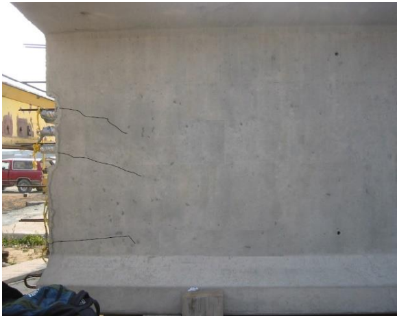
Figure 7 - Spalling cracks [6, p. 32]
