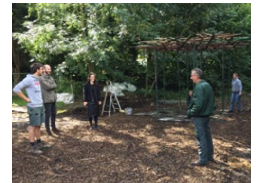
Figure 25, 26 and 27 - Materials of the local construction company and students working on site (location 2) (c) Frank Vanden Ecker - Aerial picture showing site 1 and 2.
