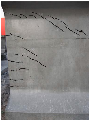
Figure 1: End zone cracks in pre-tensioned girder [1]
