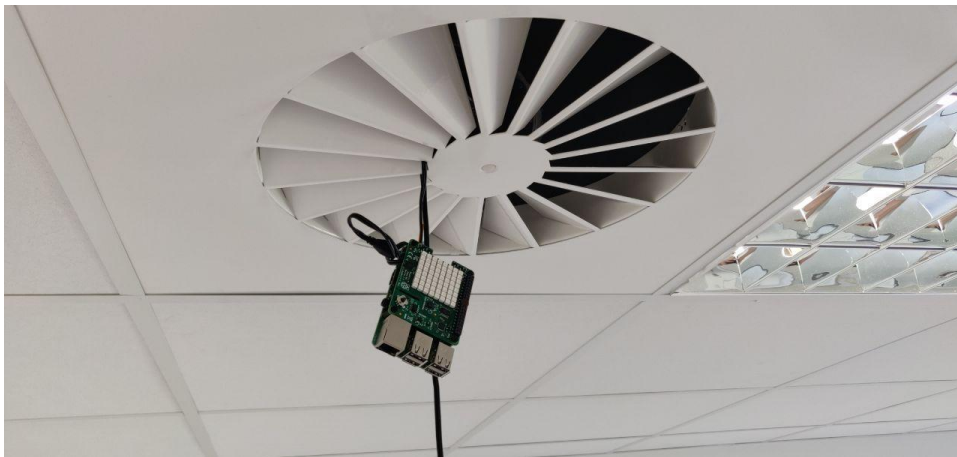
figure 7: Sensor node safely installed near the HVAC unit in the ceiling
