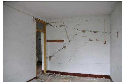
(b) Crack patter in the masonry building
