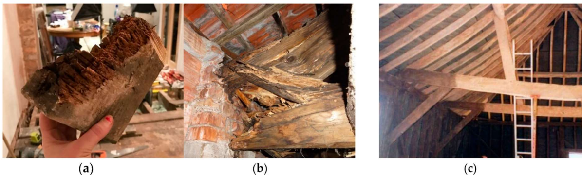
Figure 4 Examples of damage in timber structures: (a) and (b) show rotting wood at the beam ends and at the joists in the timber roof truss; (c) shows a deformed timber tie in a roof structure due to overloading [9].
