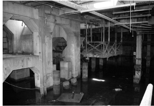
FIGURE 61 BOILER RUINS (REIMANN, 2010)
