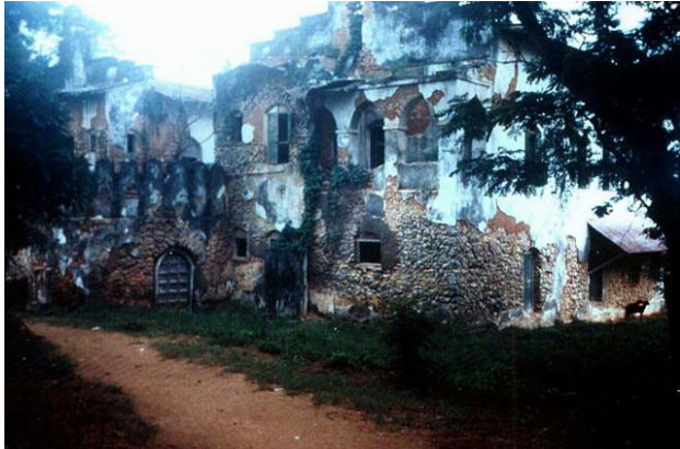
Fig 19: The building in state of despair
