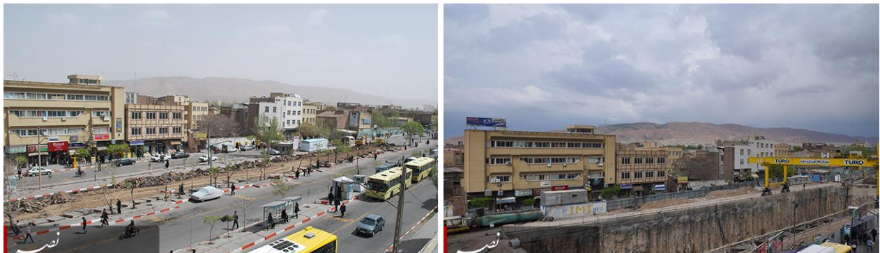
Figure 5: East Mohaqeqi bus terminal station before (left) and after (right) metro station construction works ( source )
