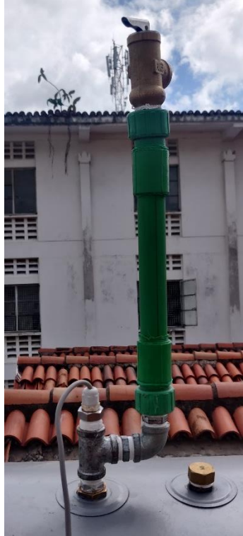
Figure 76: Temperature sensor and pressure relief valve
