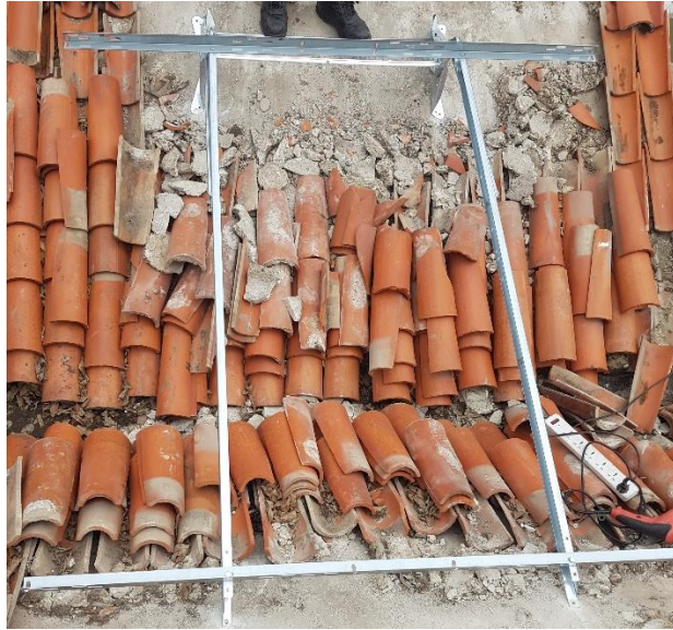
Figure 59: The support frame on the slopping roof
