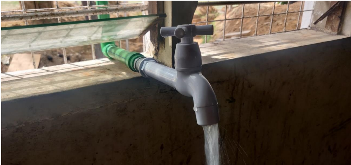
Figure 75: Hot water tap
