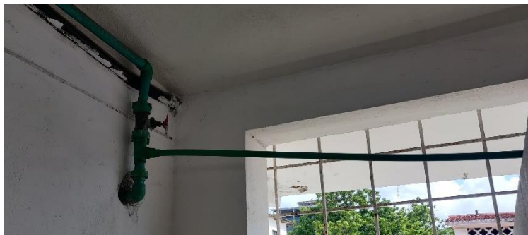
Figure 69: Cold-water pipe starting from the storage vessel
