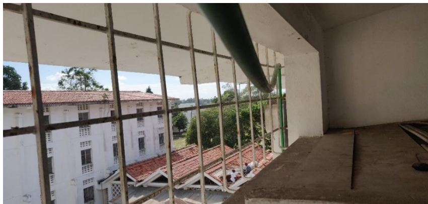
Figure 70: Cold-water pipe going outside
