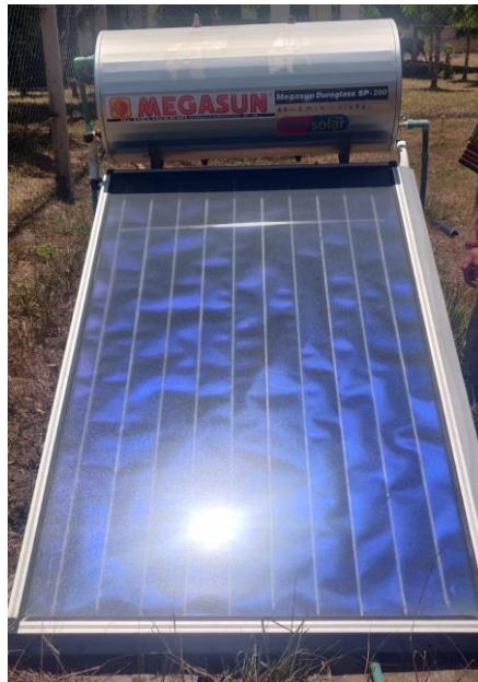
Figure 49: Solar collector installed at the MOE Mtwapa energy center
