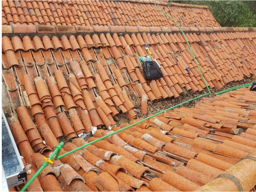
Figure 73: Start of the hot water piping
