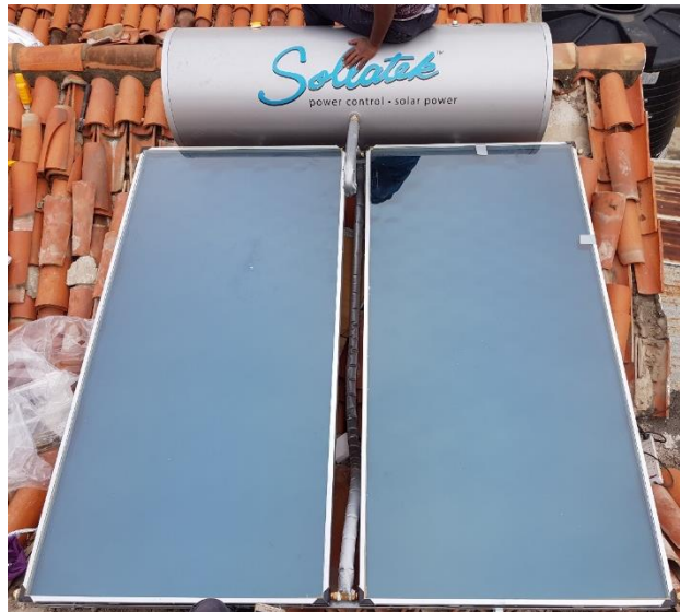
Figure 65: Storage vessel placed on the frame
