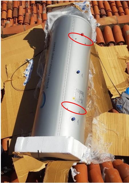
Figure 64: The water storage tank
