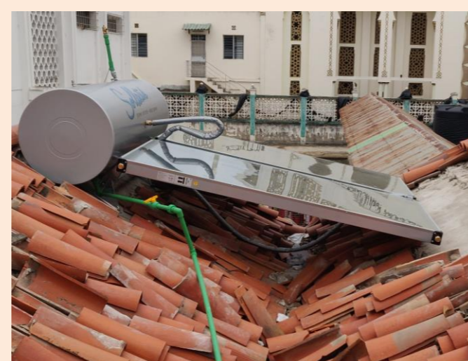
Figure 7: The solar collector on the roof, side view
