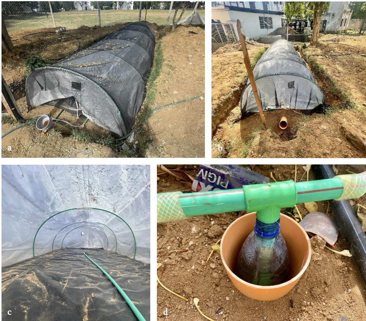
Figure 11-4: Flexi biogas installation a) front b) back c) inside of the digester d) de-watering system
