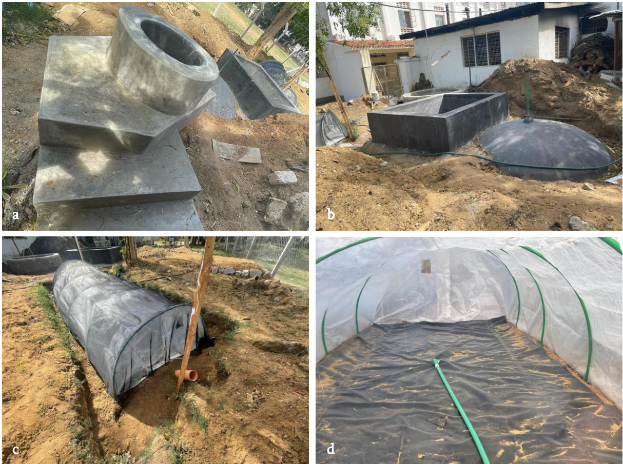
Figure 10-6: Progress of the construction: a) inlet b) fixed-dome digester c) flexi biogas installation d) inside of flexi biogas installation
