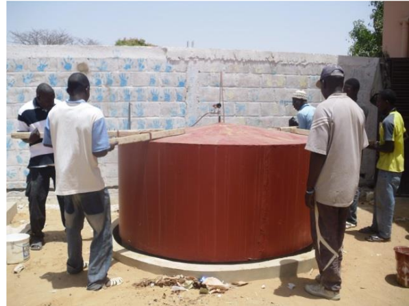
Figure 9-4: Floating-drum gasholder in Senegal
