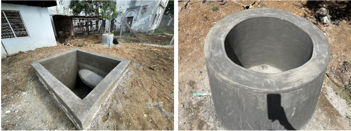
Figure 10-5: Overflow tank and inlet reservoir
