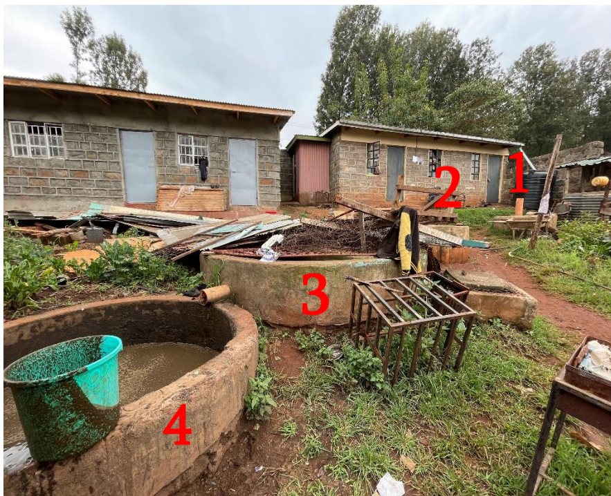
Figure 6-4: Fixed-dome installation in Dream Children's Home. 1) inlet tank 2) digester 3) overflow tank 4) digestate storage
