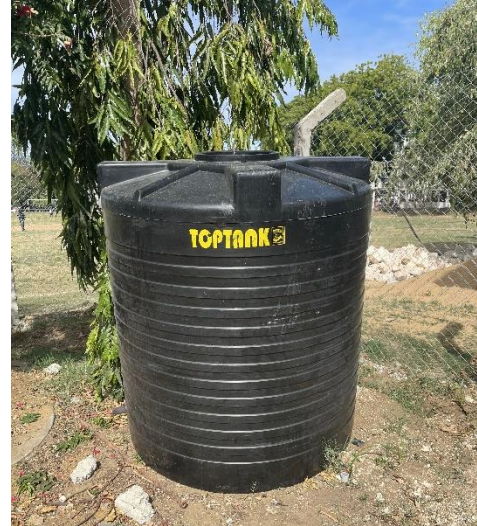
Figure 11-6 Water tank that is going to be used for the drum
