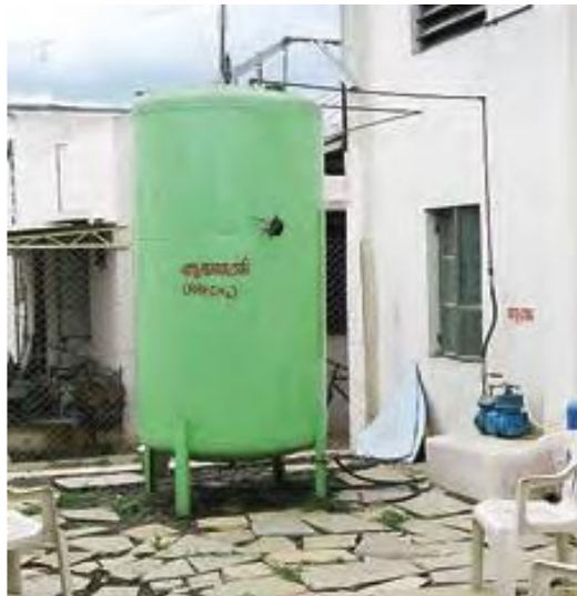
Figure 5-5: Gas storage tank with a pressure of 10 bar [9]
