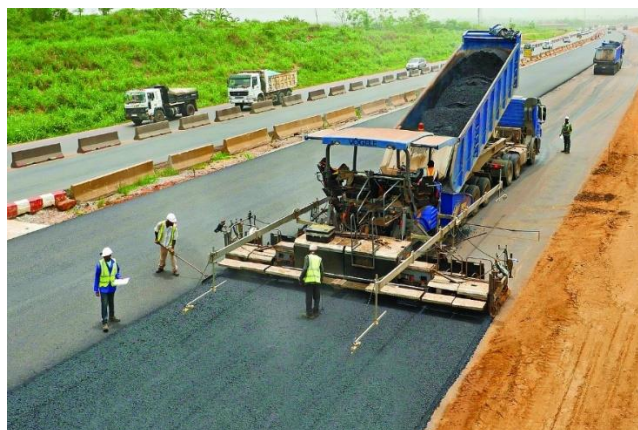
FIGURE 32 Reconstruction of Lagos-Ibadan Expressway along 'The Holy Ghost Congress' redemption campground (Julius Berger, 2019).
