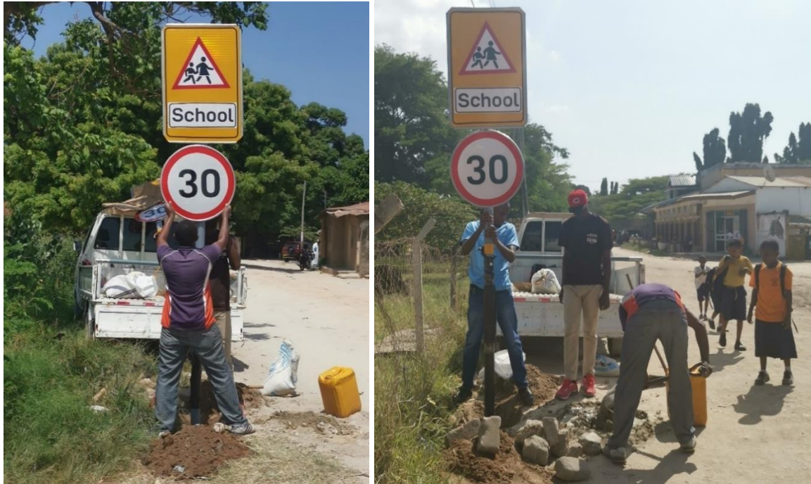
FIGURE 28 School zone and speed limit sign Installation at the beginning and end of the SSZ.
