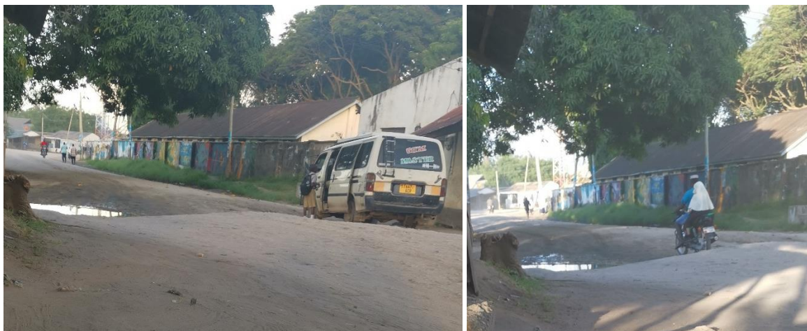
FIGURE 30 Pothole on the road alongside Kigamboni P.S.
