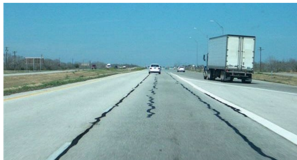
Figure 1: Longitudinal or top-down cracking [1]
