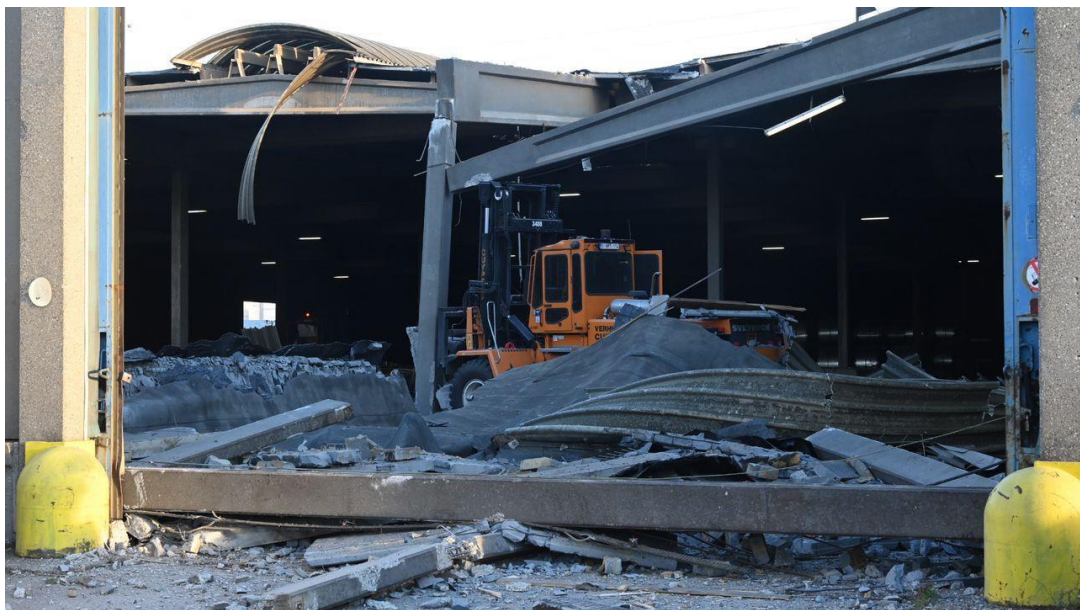
Figuur 3: Ingestorte loods in Antwerpse haven [4]
