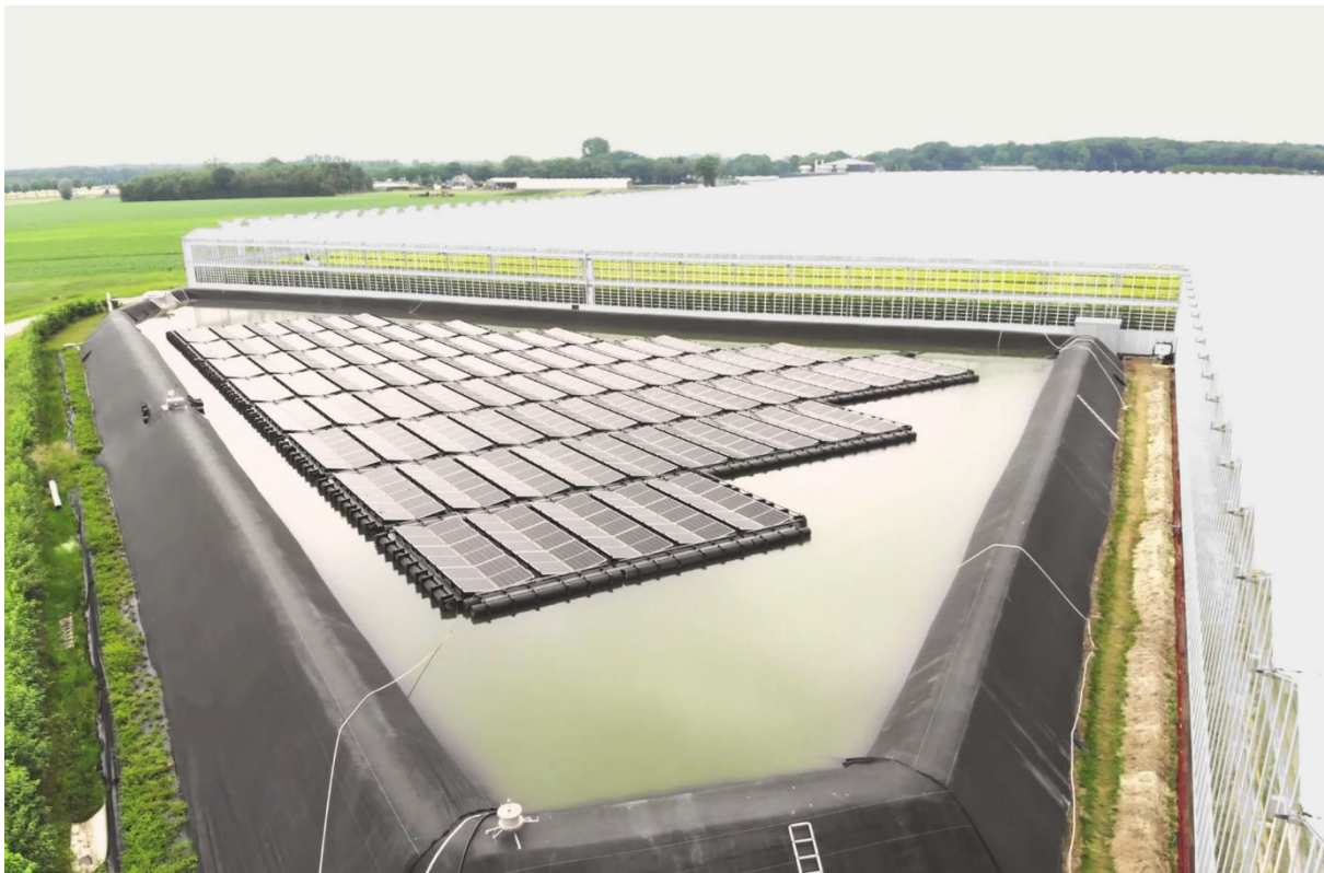
Figure 18: Aerial photo of Clicfloats FPV plant [40]
