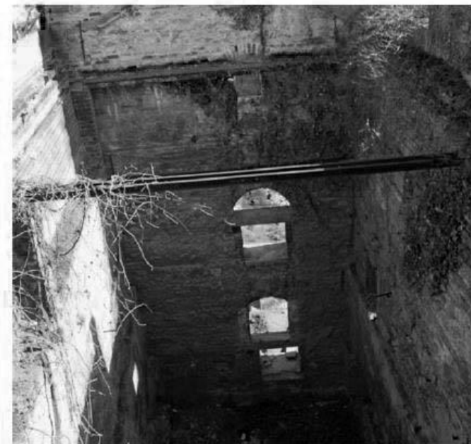
Figure 25 - The current situation of the roof of the mill from the warehouse
