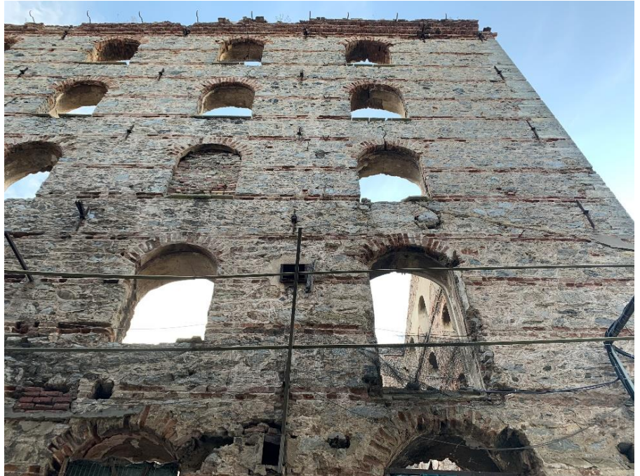
Figure 28-Picture from 2022, showing the deteriorated roof invaded by plants. The metal carriers of the wooden flooring
