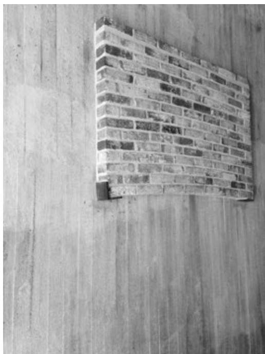
Fig. 7.11 Masonry detail, St. Mark's Church, Bjorkhagen Sweden, 1960. Experimenting with deformation from a straight to a vaulted expression. © Steven Schenk.
