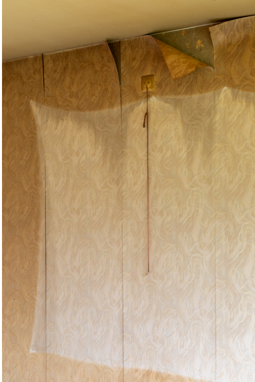
Fig. 2 Interior detail in the northern blocks. The yellowed wallpaper with the white void – a trace of its former inhabitation – is peeling. © Elisabeth Broekaert, 2020.
