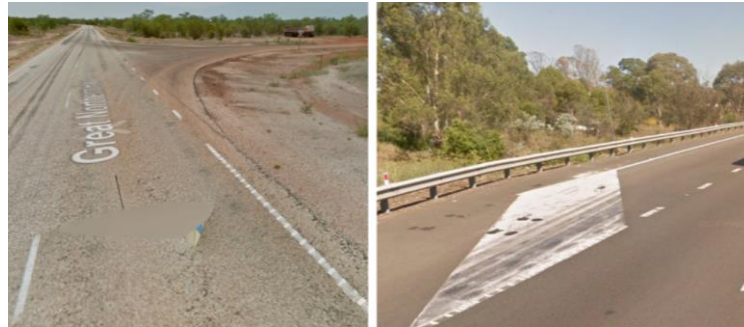
c) Example of obscure intersection and exit ramp
