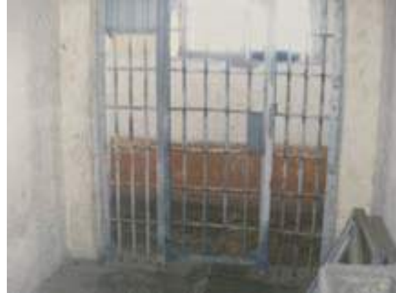
Figure 32 Looking towards the hallway from inside of a cell. It had no access to sunlight and was closed up as shown in fig. 33. (Kalan Mühendislik, 2008)
