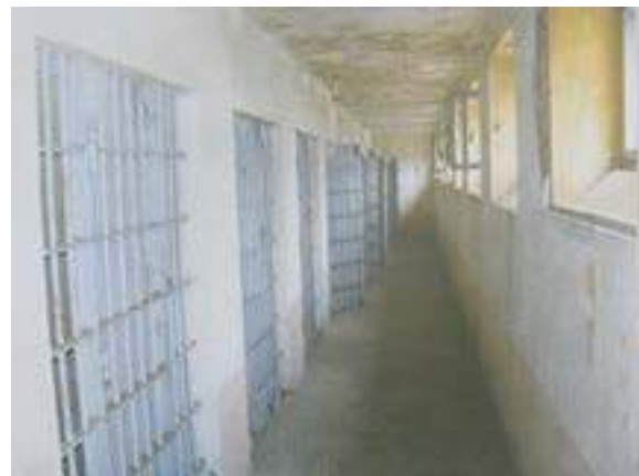
Figure 34 The hallway in front of the cells of the northern facade. (Kalan Mühendislik, 2008)
