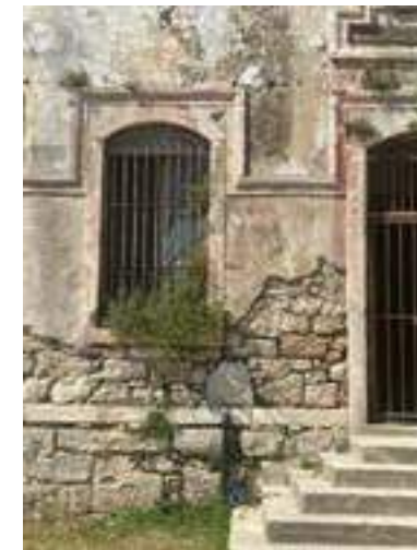
Figure 23 This is the front facade of the Youth Detention Centre. An example of efflorescence and spalling.
