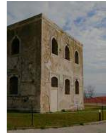
Figure 25 The western facade of the detention centre shows us the moisture-water problems.
