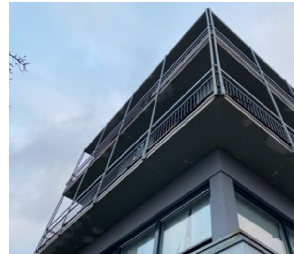
Fig. 4.2 Pand Mooren in current state [the decay, dated 17-12-2022.
