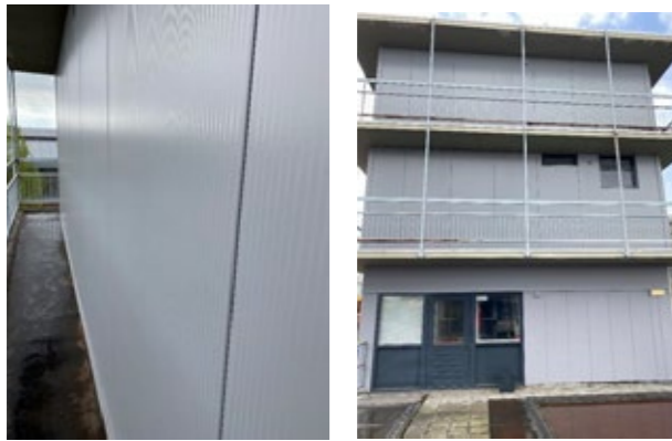
Fig. 4.3 The recently installed sandwich panels in the upper two levels. Own pictures dated 25-4-2023.
