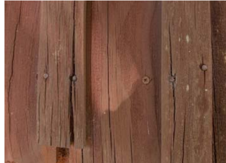
Figure 4. Example of cracks
