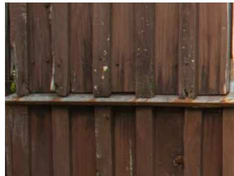
Figure 6. Example of sill failure
