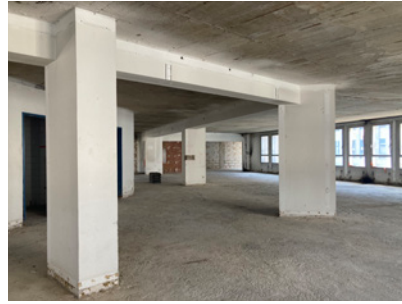
Fig. 16: Current interior view of a typical floor level, showing how much space is taken up by the central core and awkwardly-placed structural columns, reducing the useable floor area. Photograph by the author.
