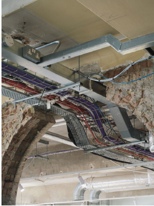
Fig. 5: Cable tray running straight through an existing brick arch, uncovered during the stripping back of Southover House. Photograph by Henry Woide. Courtesy of Material Cultures.
