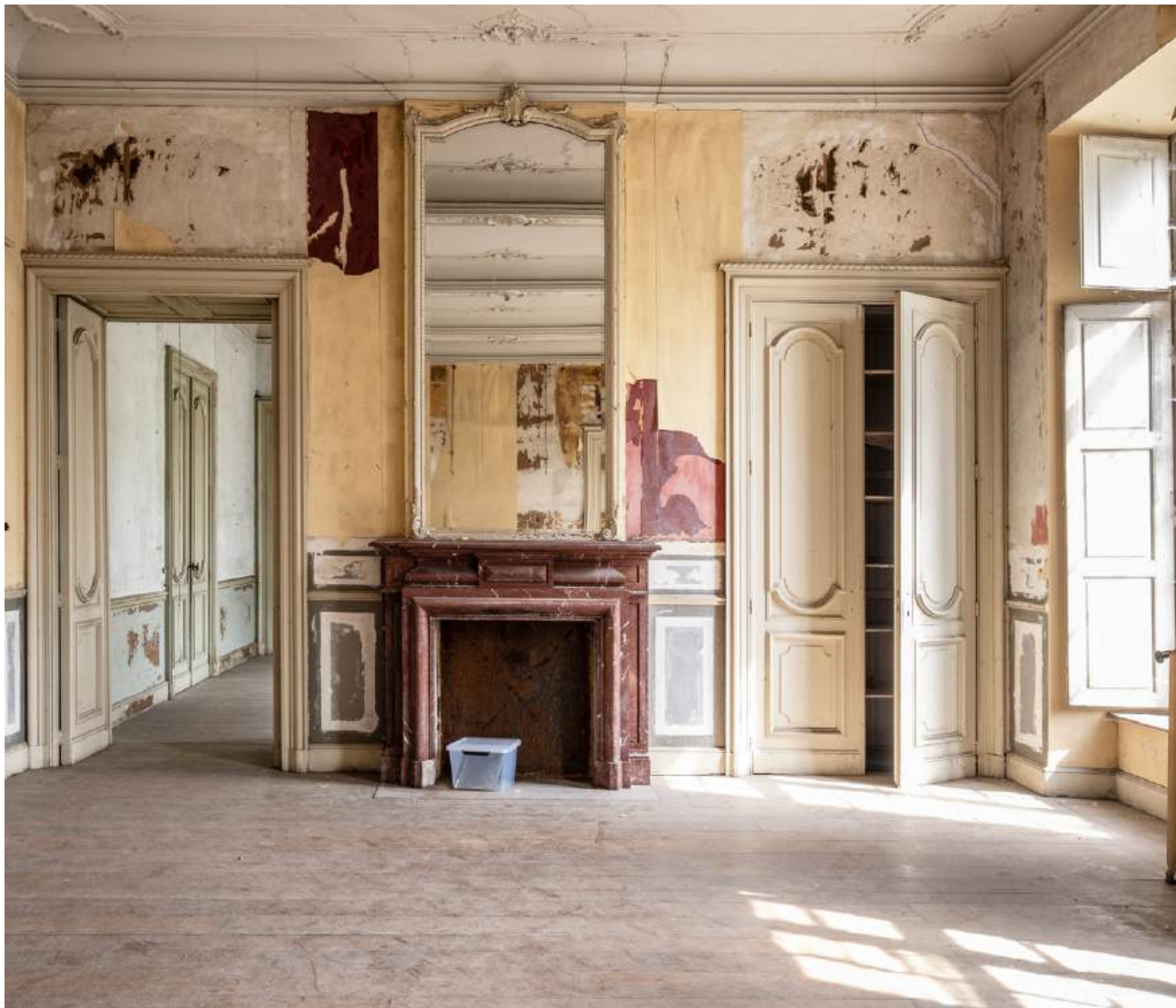
Figure 1.1 Ruinous condition of former dining room.
