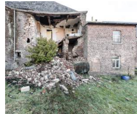
Figure 3.12 Collapsed brick wall.
