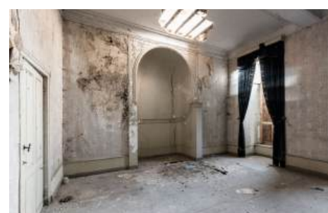
Figure 1.10 Plaster detaching from walls and ceiling.
