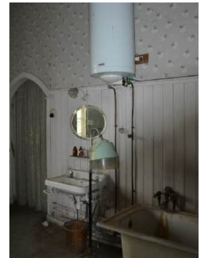
Figure 3.28 Outdated plumbing system.
