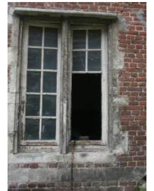
Figure 3.14 Broken window glazing.
