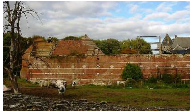
Figure 1.11 Structural collapse of the farm building.
