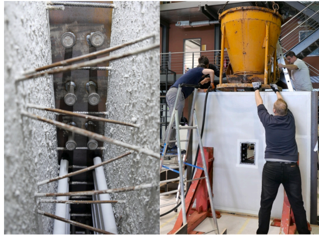
(d) View from the inside of the wall (pre-casting) and on-site casting of the concrete infill
